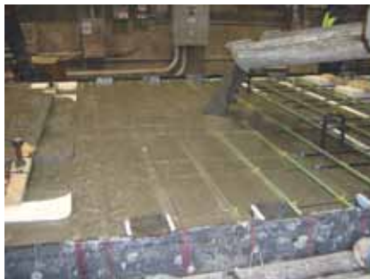
On the 24th Street bridge, the full-depth precast concrete panels were fabricated in a manufacturing plant using self-consolidating concrete.
