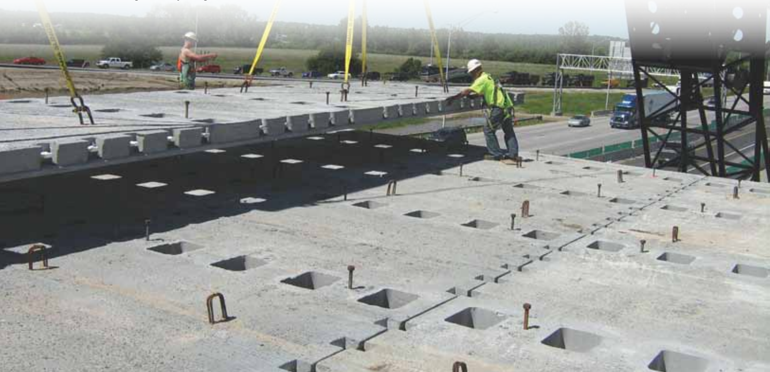
A full-depth precast concrete deck panel is installed on the 24th Street bridge over I-29/I-80 in Council Bluffs, Iowa, the first Highways for LIFE project in that state. All Photos: Iowa Department of Transportation.
