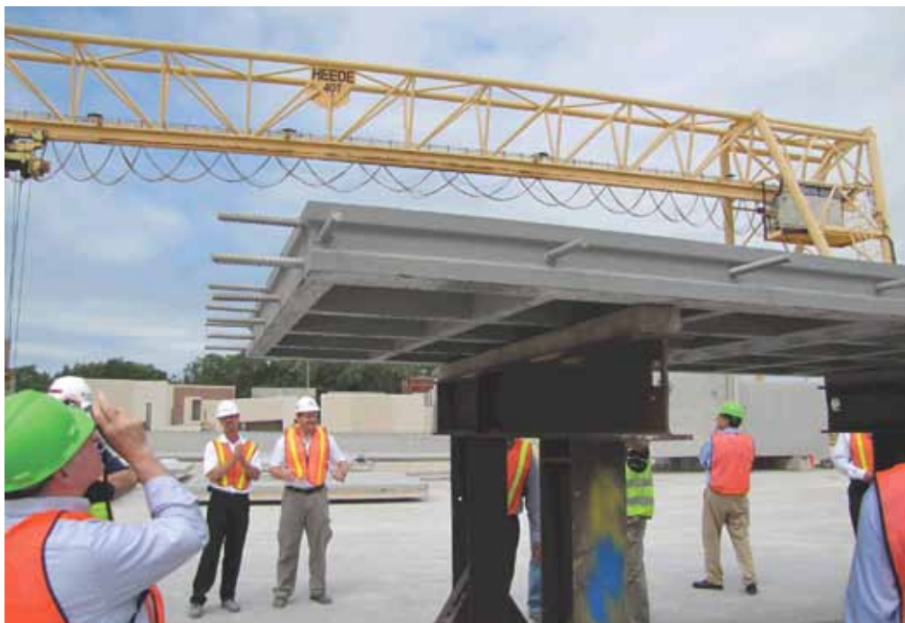
A Highways for LIFE project is the Little Cedar Creek Bridge in Wapello County, Iowa. A two-way ribbed deck panel of ultra-high-performance concrete (UHPC) will be grouted to the girders with UHPC. The panel is 8-in. deep with a top flange 2 1/2-in. thick. It weighs one-third as much as a typical deck panel. The panels attained a concrete compressive strength of 29,000 psi. They were on display at a FHWA showcase at the Coreslab Structures Inc. plant in Omaha, Neb.
