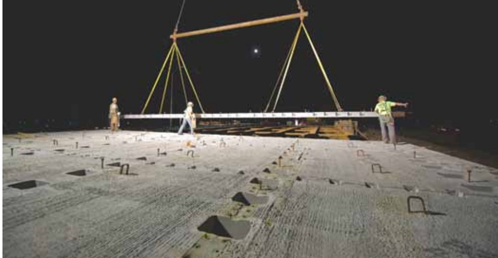
Work on the 24th Street bridge included nighttime installation of precast concrete panels over the traveled lanes in order to minimize traffic interruption.
