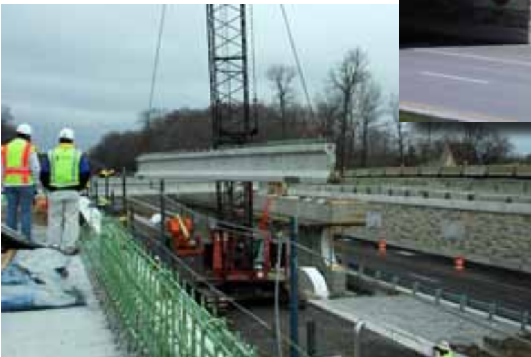
Each of the bridges' framing consists of 15 beam lines, with the 11 interior beams parallel to each other and each of the outside two rows of beams splayed to fit the copings. Photo: American Structurepoint Inc.
